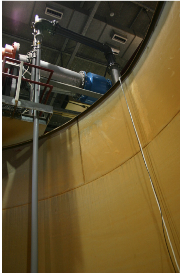
Fig. 7. Cantilever plastic pipe in the dry tank.
